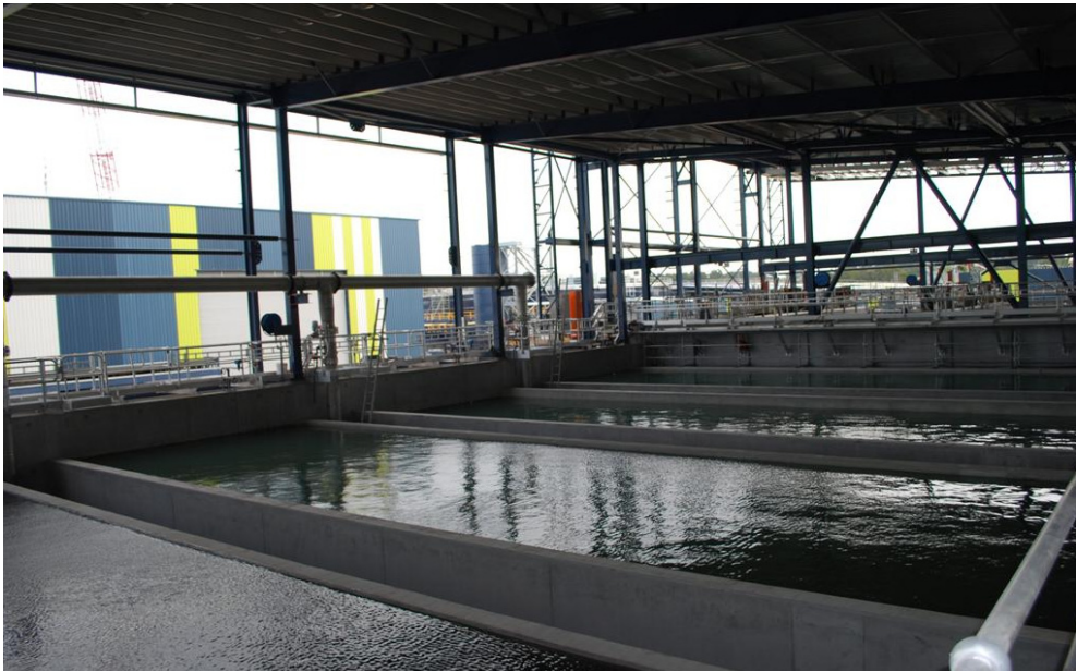
Fig. 25. Gravity dual media filters (Australian desalination plant)
