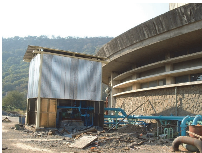
Fig. 4. Desalination unit located outside Cirus annulus area
