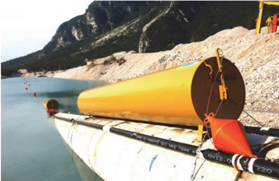
Fig. 2. Launch of a submerged methane pipe. The buoys along the launched length are in full view.
